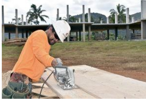
Donald Pacol of McClone Construction Company rips lumber for forms for the Timbers Kauai Ocean Club and Residences' second building, Tuesday afternoon at Nawiliwili.
